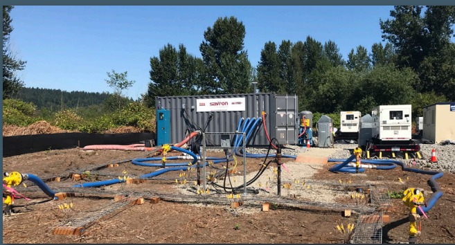
IMAGE 1: PDE test area showing the ignition / air injection well, associated thermocouple network, the STAR control trailer, and auxiliary equipment.
