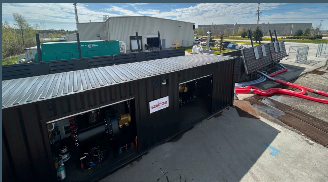
IMAGE 1: STARxpress plant at Savron's Boxwood facility consisting of a control/equipment container (foreground), two 35 m 3 vessels with retractable roofs (one vessel shown to the right, with the roof of other visible behind the control container), and associated connections.
